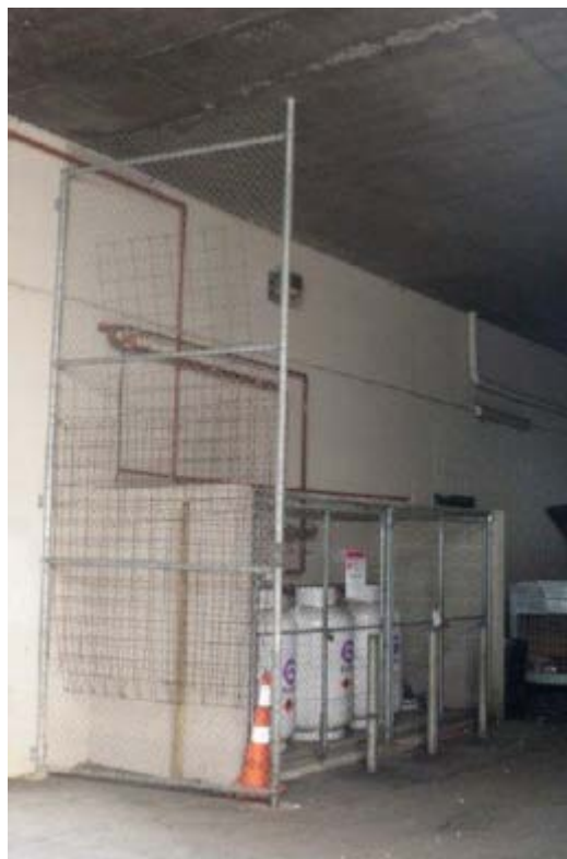
The 220 kg cylinders dwarfed in the blocked service area.
