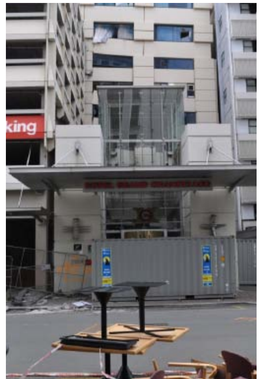
The slump of the hotel is evident in the windows.
